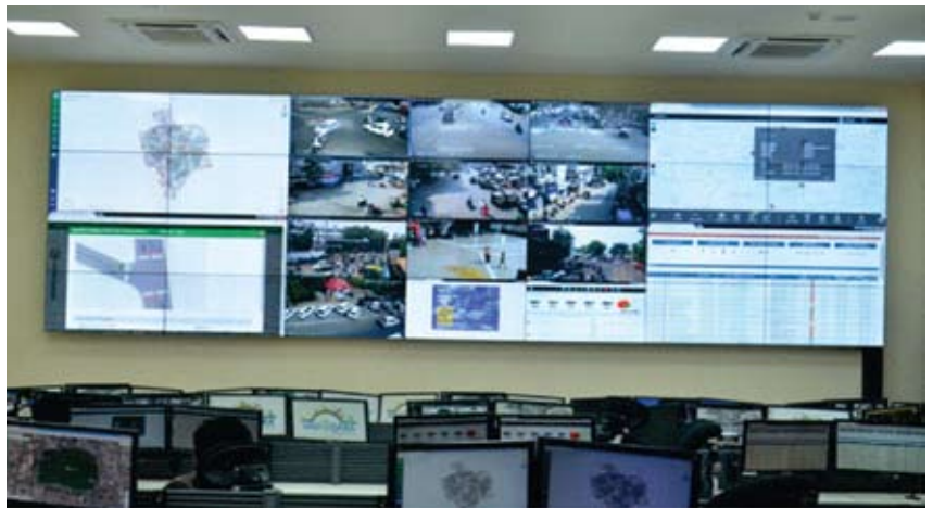
Integrated Command and Control Center at Vadodra
