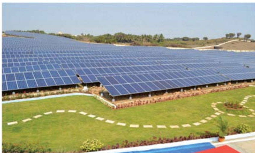
Solar PV Installation, Diu Smart City
